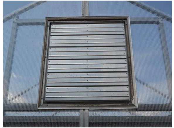
Figure 2: Motorized power shutter installed (outside).
